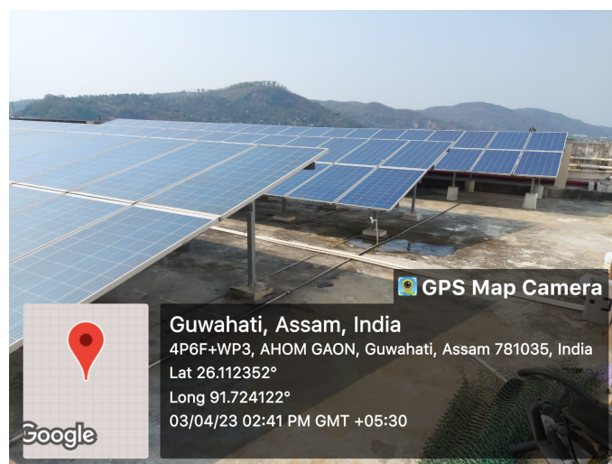
Solar Panels installed on the terraces of Blocks A, B, C and the Harsha Hostel of the university.
